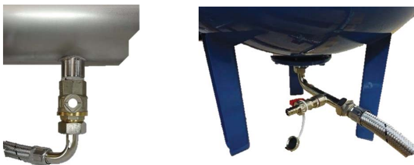
Fig. 1.7a & b Isolation valve on system pipework & Drain cock on vessel
