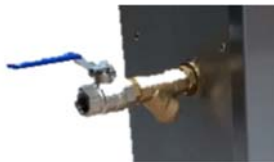
Fig 2.2 Mains water inlet isolation valve & strainer
