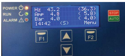
Fig 2.1 Controls/display (1 per pump motor)
