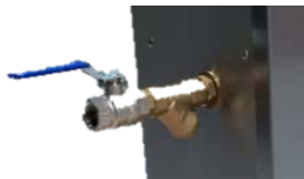
Fig 2.2 Mains water inlet isolation valve & strainer
